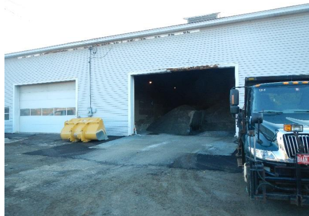
Photo 2: Roof drains onto parking area with high sediment and salt loads
