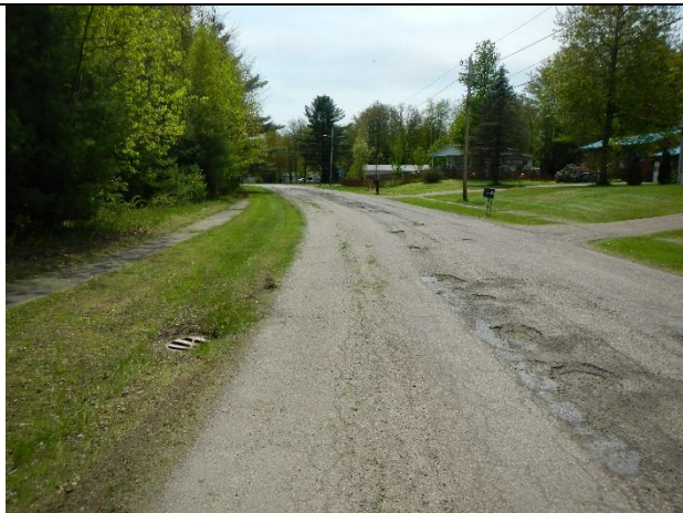
Photo 1: Potholes and pavement damage in low point of road at catch basins.
