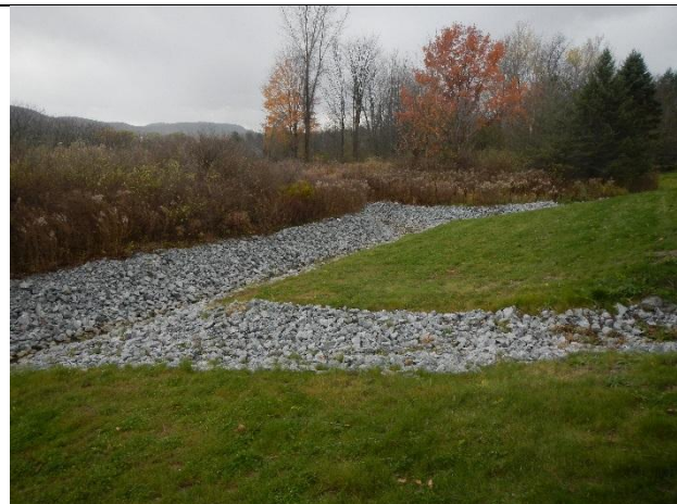
Photo 2: Outlet from wet pond draining to the southern end of the stone lined swale.
