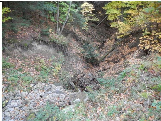
Photo 1: Large and active gully at the outlet of the Stacy St storm drainage system
