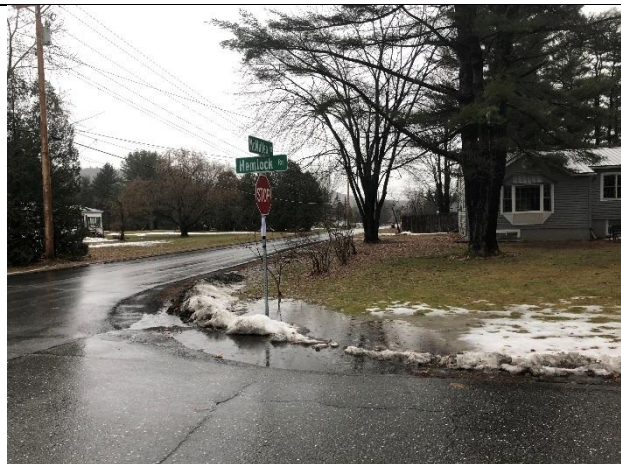
Photo 2: Ponding 6" over dry well during a small runoff event
