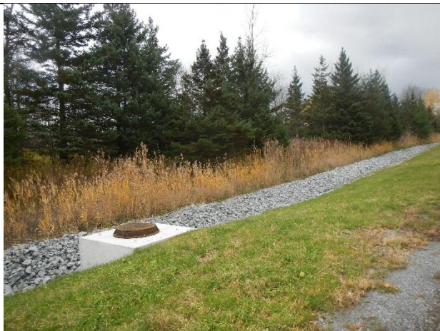
Photo 1: Northeast end of stone swale and outlet structure with overflow from wet pond.
